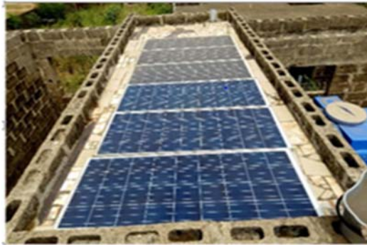
Figure 4: The solar panel as installed
